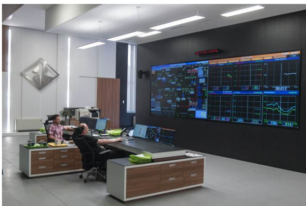
Figure 5: Command and control centers (JPEP BiH - NC)
