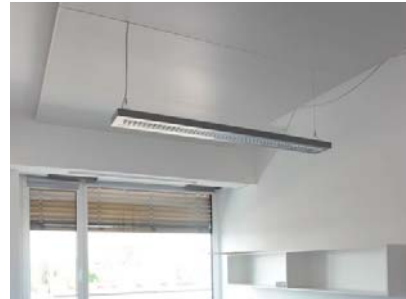
Figure 5. Heating/cooling ceiling panels in refurbished offices.
